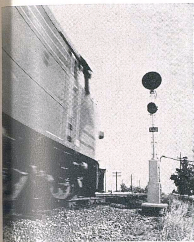
SERVOSAFE® Hot Box Detective* here signals train crew automatically, if overheated journal bearing is detected on passing freight at remote spot on main line.
